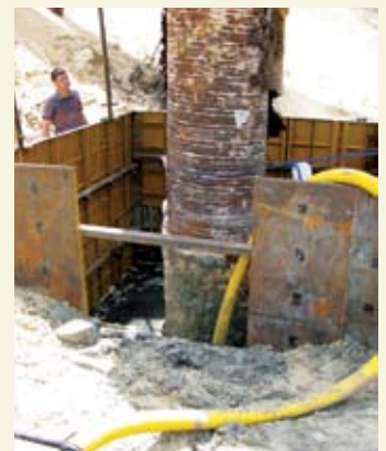
The extent of the damage to the pier and commencement of construction of the temporary working chamber.
