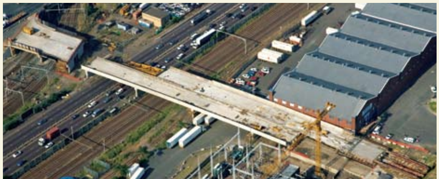
The incremental launch of this bridge is taking place above the busy Metrorail lines serving the south of Durban.
