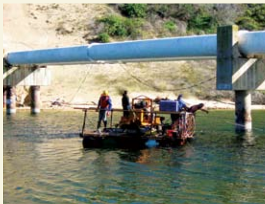
Members of the team move the temporary working platform into position under the center piers of the pipe bridge.
