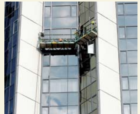
The existing structure would not have been able to take the weight of conventional scaffolding.
