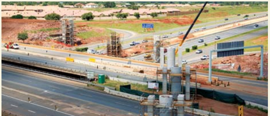
An aerial view of construction underway, showing the piers and the curve the road surface of the bridge will follow.
