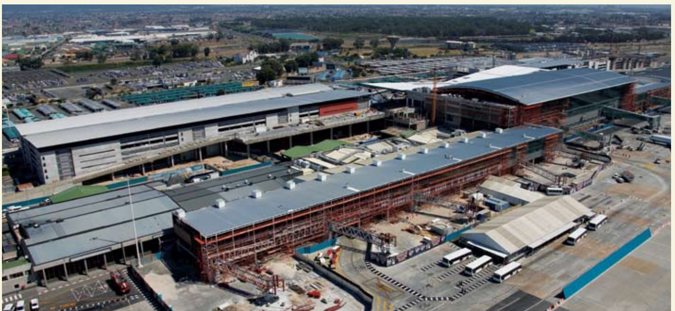
An aerial view of construction progress at the CTIA, with the multi-storey carpark in the forefront.
