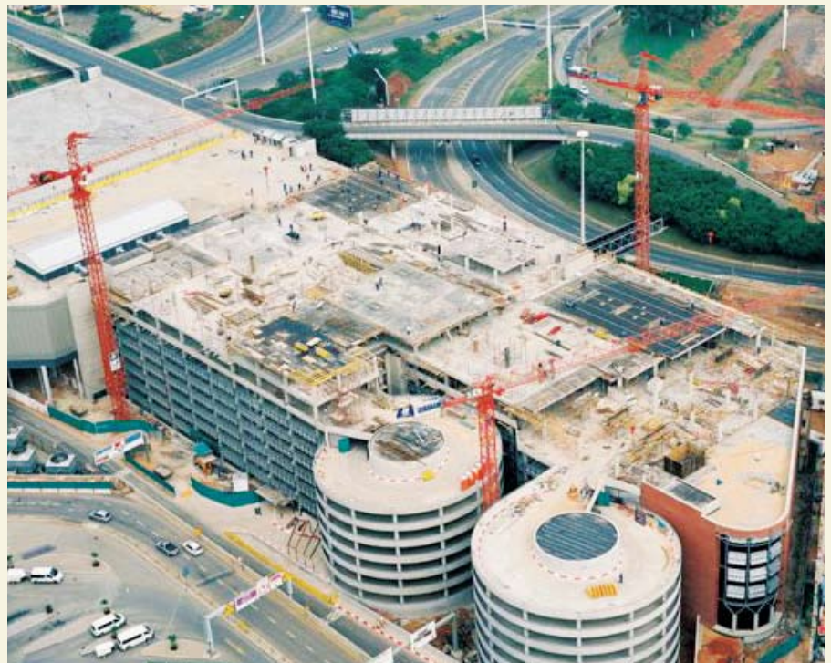
An aerial photograph of the multi-storey carpark with the two landmark ramp towers, with the Gautrain bridge visible on the northern side of the building. Construction of the hotel has commenced on the roof of the carpark, behind the ramp towers and to the left of the Gautrain bridge.
