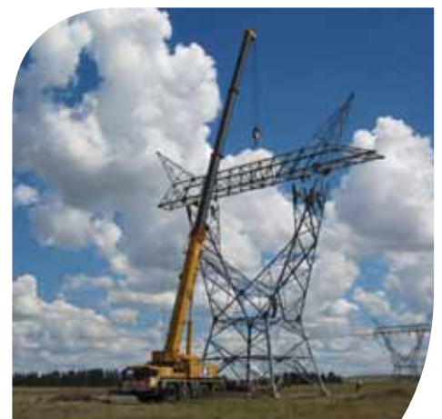
The erection of the 400 kV tower on the Majuba turn in, using a 90 ton crane.
